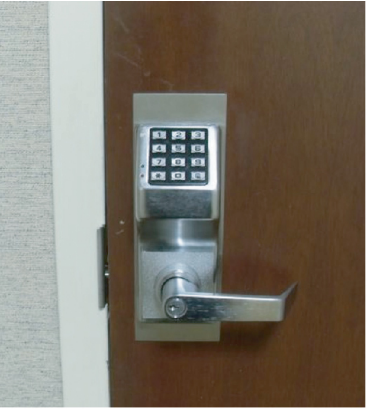
Access Controlled Door
